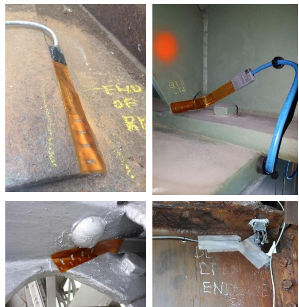
Figure 2 Sensor deployment examples on various bridges ranging in construction date from 1883 to 1971. Sensor installation is performed on top of existing coating, and can also operate in the presence of corrosion.
